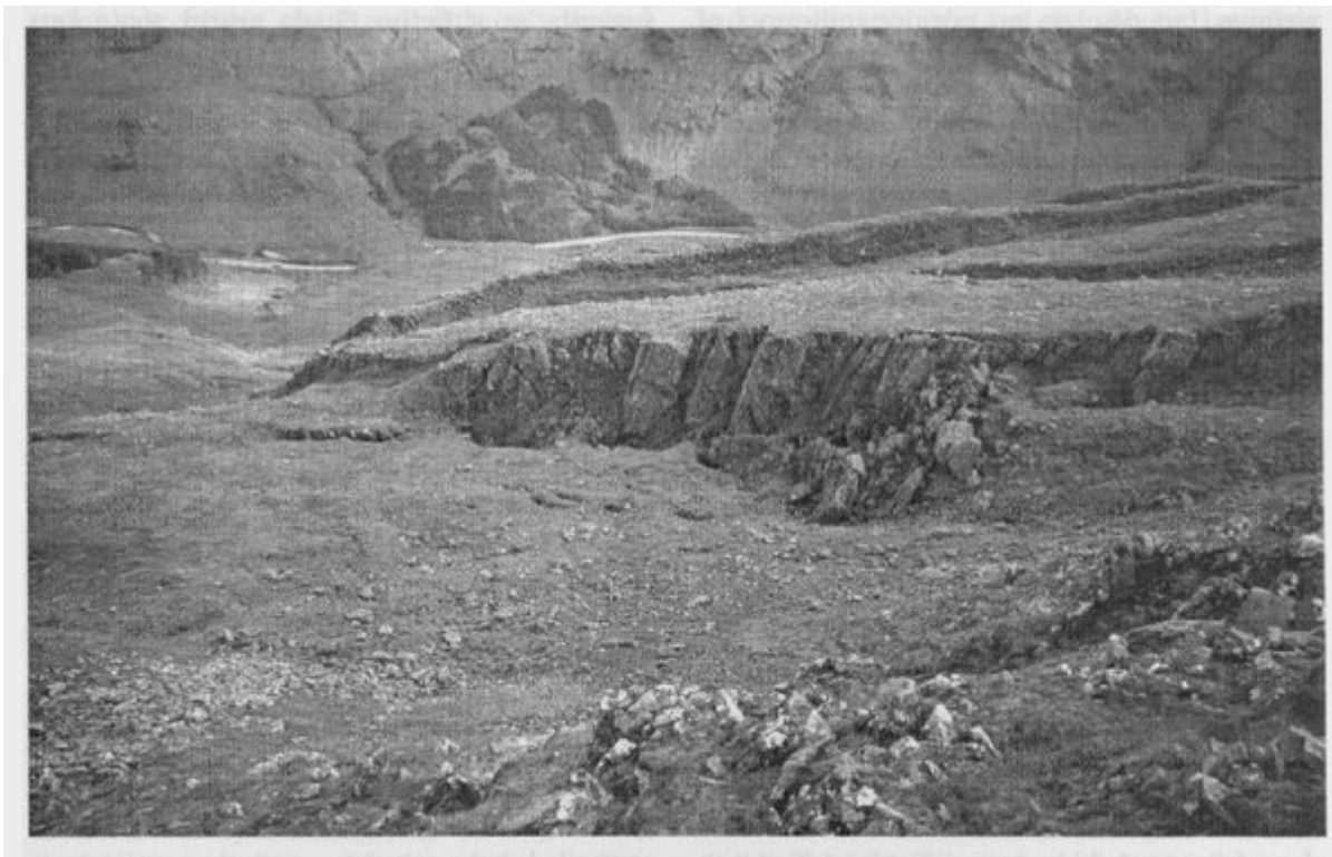
(Figure 2.27) Antiscarps and graben wall below the summit (Zone D). The bulging toe (hiding the road) creates a local gorge. The slide cavity with fissured debris-mass can be seen in the foreground. The long parapet/ antiscarp and uphill-facing crag are marked on (Figure 2.24). (Photo: D. Jarman.)
