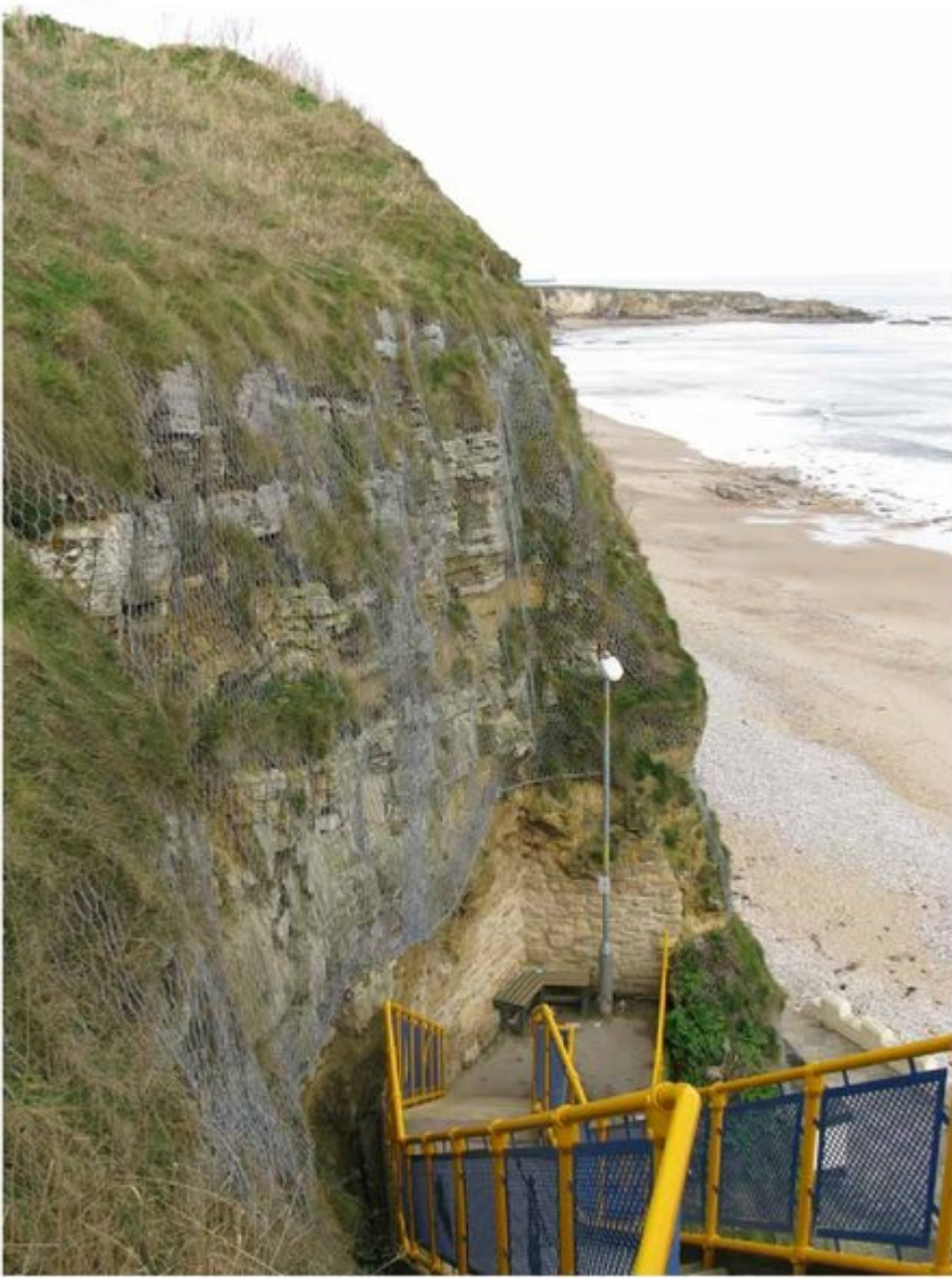
(Plate 13) Wire mesh protection of the cliffs near the steps at Marsden Bay. The nature of the rocks can still be seen through the stabilisation measures (February 2009).
